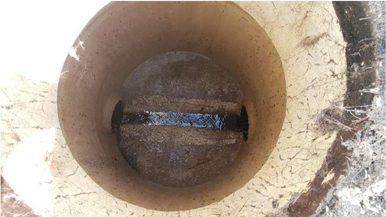
2. East PLCT MH-9 invert.
