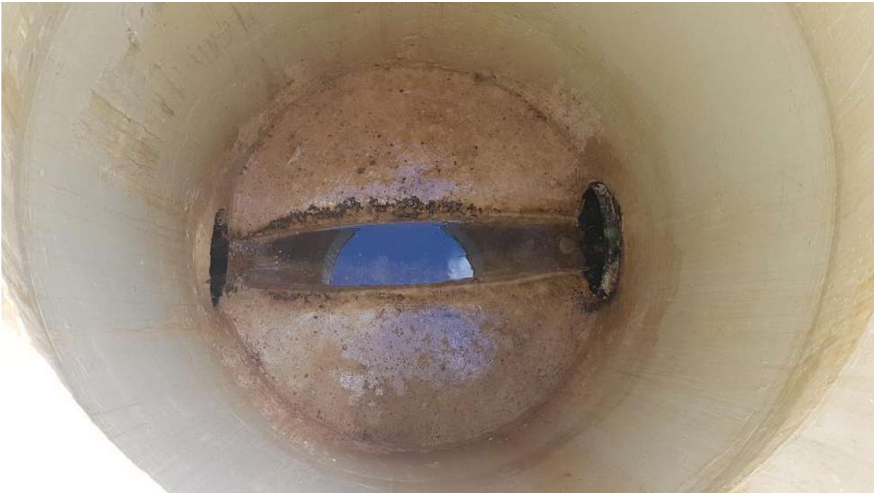
4. West PLCT MH-11 invert.
